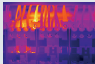
Maintain systems: Identify excessively high temperatures in circuit breakers and electrical components before breakdowns can occur.
